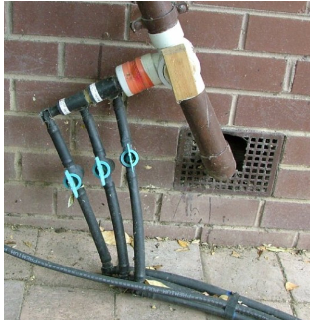
The diverter manifold
